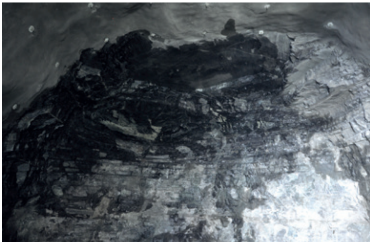
Figure 9: Rock mass exposure at the tunnel face of Skarvberg tunnel, outside the failure section shown in Figure 2a, with clearly well-defined lamination in metasandstones, and some roof delamination. Photo: E. Skretting (2020).
