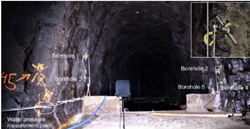
Figure 4. Location of boreholes in the tunnel looking upstream and a detail (top right corner).
