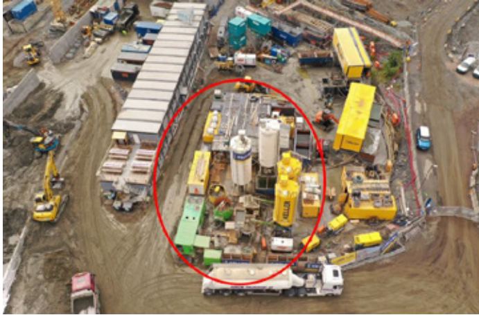
Fig.9: Site setup: mixing station for 2 jet grouting units (red circle) and backflow treatment plant, on the right side the single entrance to the site can be seen
