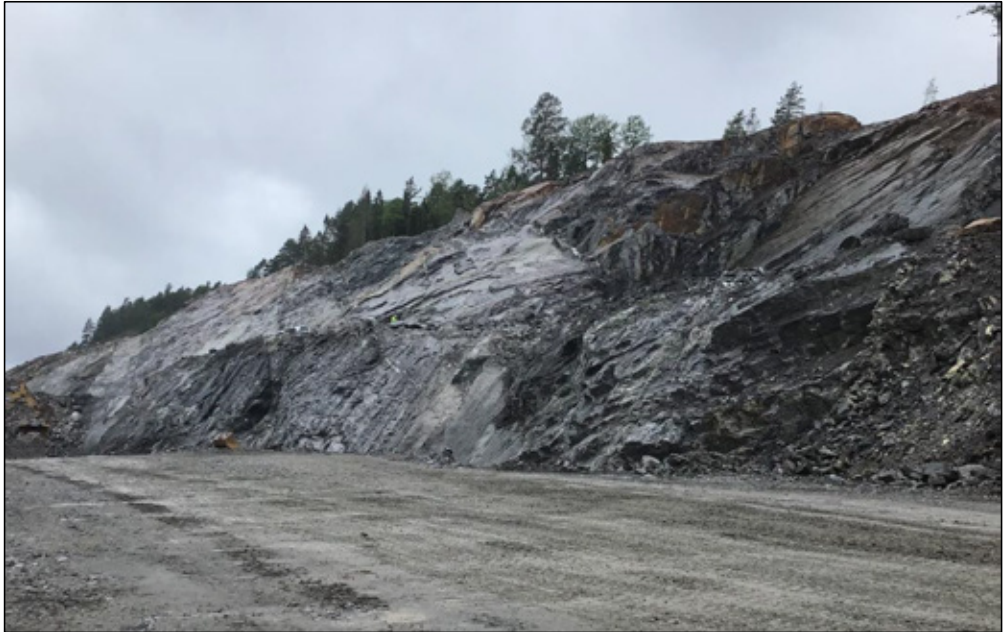
Fig 2 A portion of 15330-16360R showing surface of pervious planar slide along the foliation surface in the top right corner.
