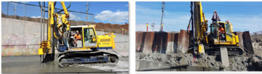
Fig.10: Left is the double axis jet grouting rig and right the single axis rig executing the soil improvement works
