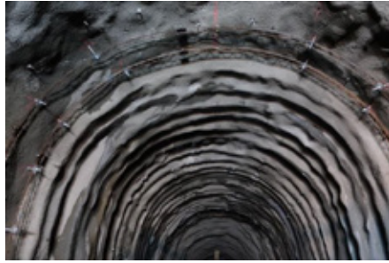
Figur 9: Tung sikring under Alnaelvtunnelen.
