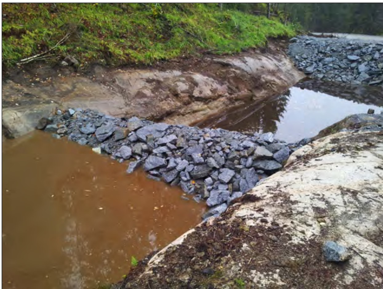
Figure 1 A double camber semi permeable sedimentation pond
