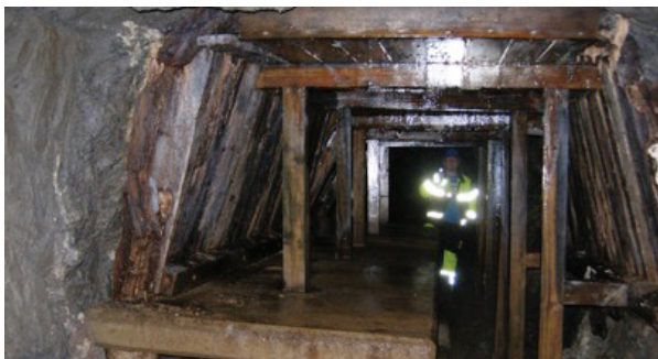
Emma Hjort tunnel for fresh and drain water pipes – timber support – although in poor condition, parts of the timber supports are still intact after more than 50 years in operation
