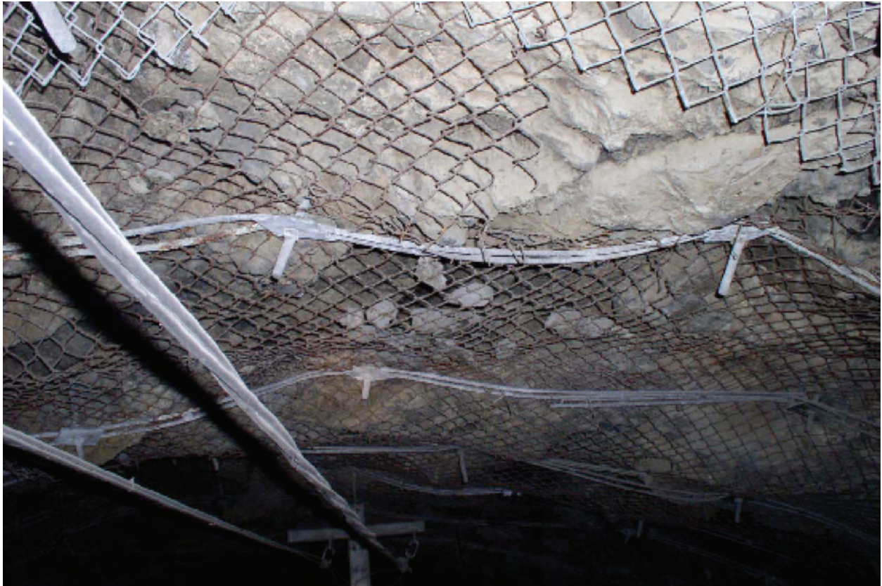
Figure 2: A 25-year-old wire mesh, completely corroded. An attempt has later been made to repair the damage using new wire mesh and steel straps.
