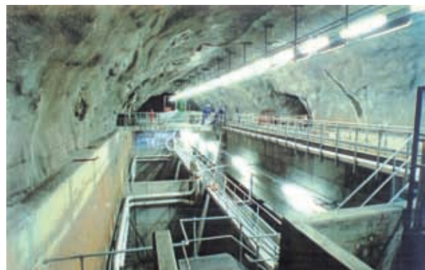
VEAS waste water treatment plant, from one of several caverns.
