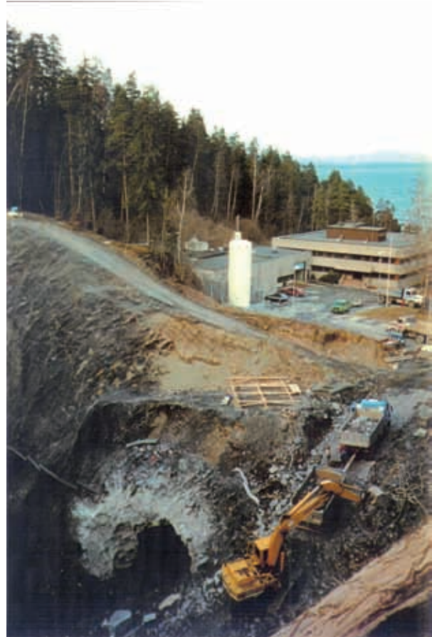
VEAS waste water treatment plant west of Oslo
