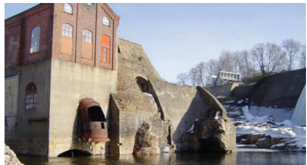
Before the cofferdam was constructed, the old tailrace tunnel at Borregaard hydropower plant was filled with water
