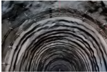
Figur 9: Tung sikring under Alnaelvtunnelen.
