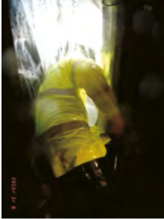
Photo 3 Major water inflow to the TBM excavation chamber
