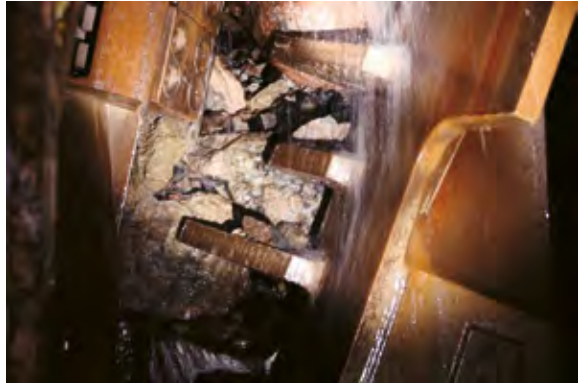
Photo 4 Highly weathered gneiss caused flowing ground over and behind the shield that blocks the cutterhead
