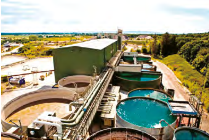
Photo 5 Slurry Treatment Plant (STP) on the Hallandsås Project ensures correct treatment and release water coming from the tunnels
