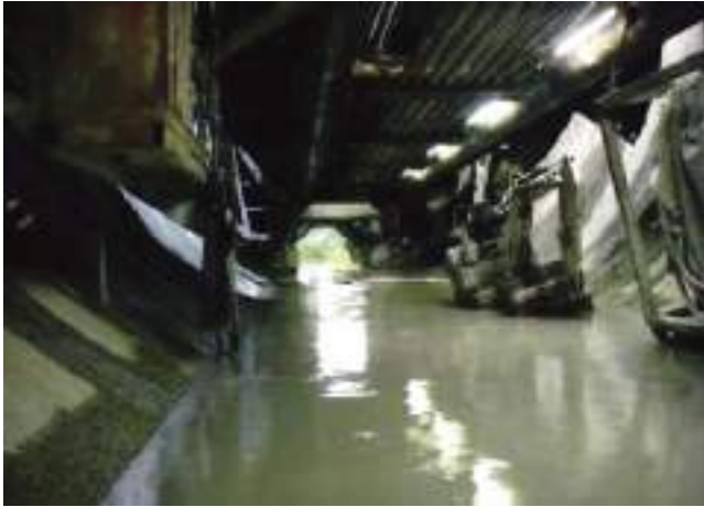
Figure 19: Inrush of water in the East Tube
