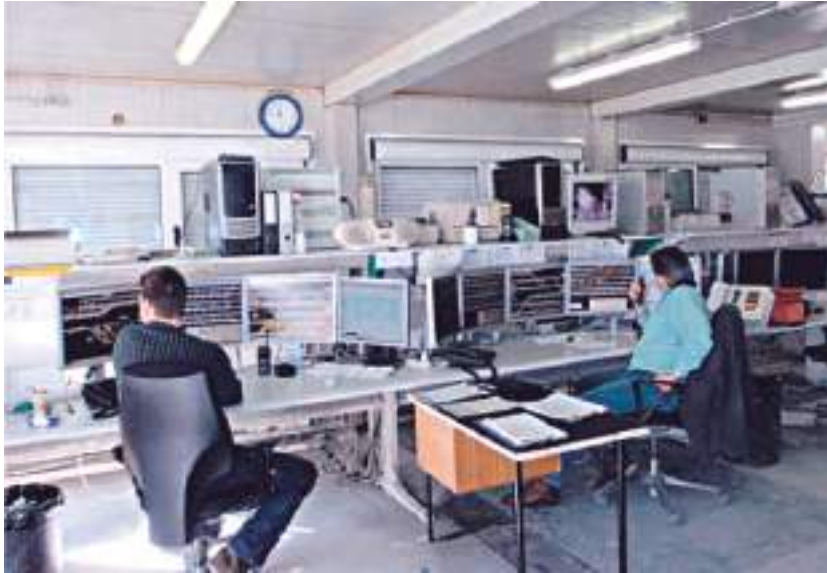
Figure 7: The central train control facility at the Bodio work yard
