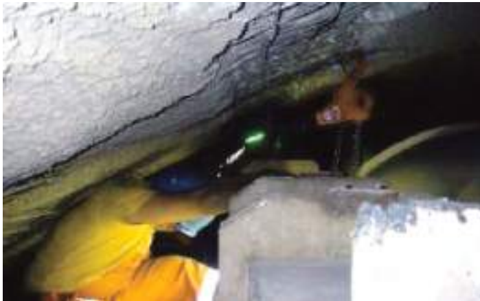
Figure 12: Back-up installation – deformation
