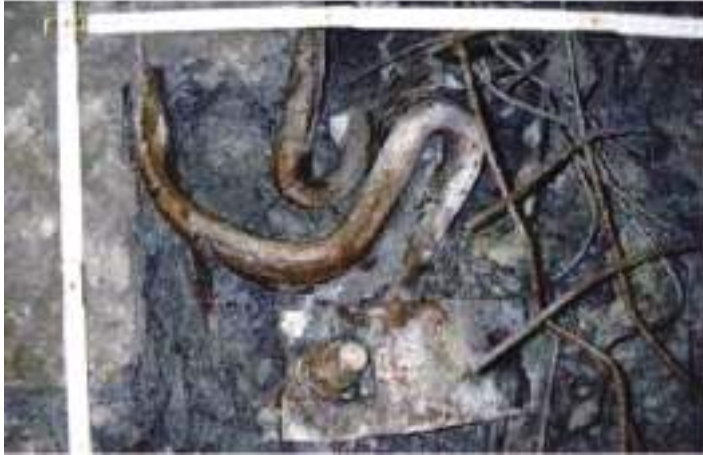
Figure 10: Deformed steel arch, eastern tube
