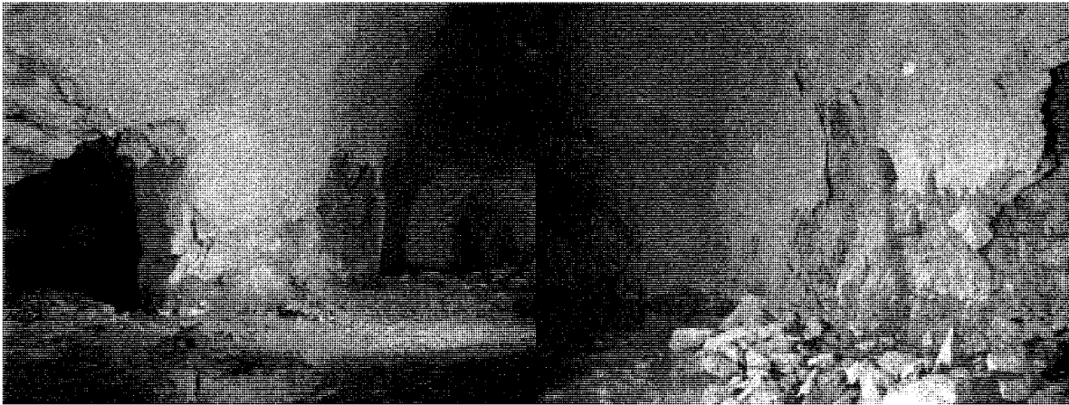
Figure 20. Spalling in the distributor tunnels
